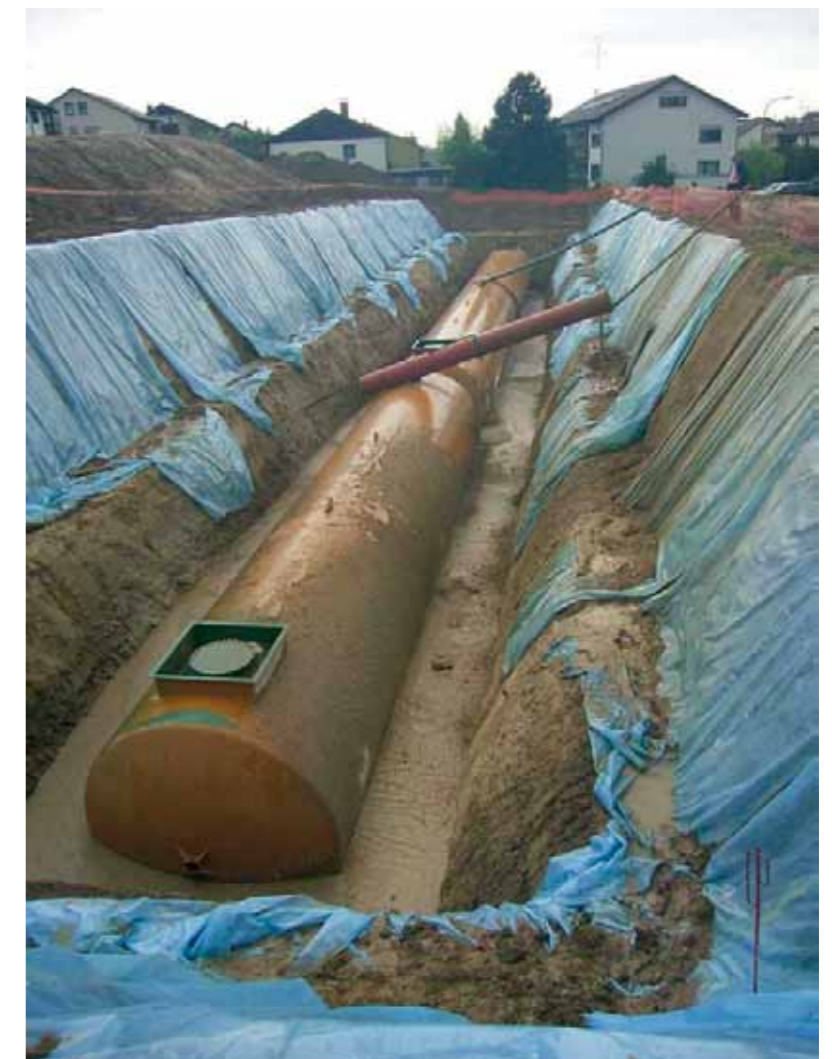
Rainwater storage tank :
